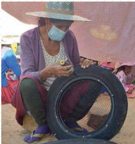
Figure 7. Construction of window frames made from tires. Source: Hábitat para la Humanidad Bolivia, 2021
